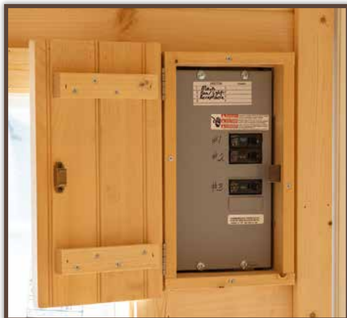
Breaker Box with Breakers
